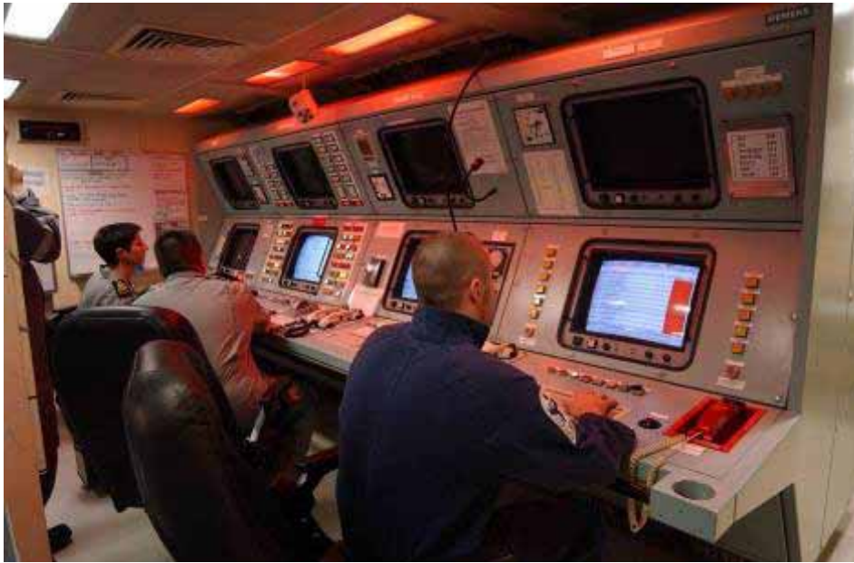
Machinery Control Room
